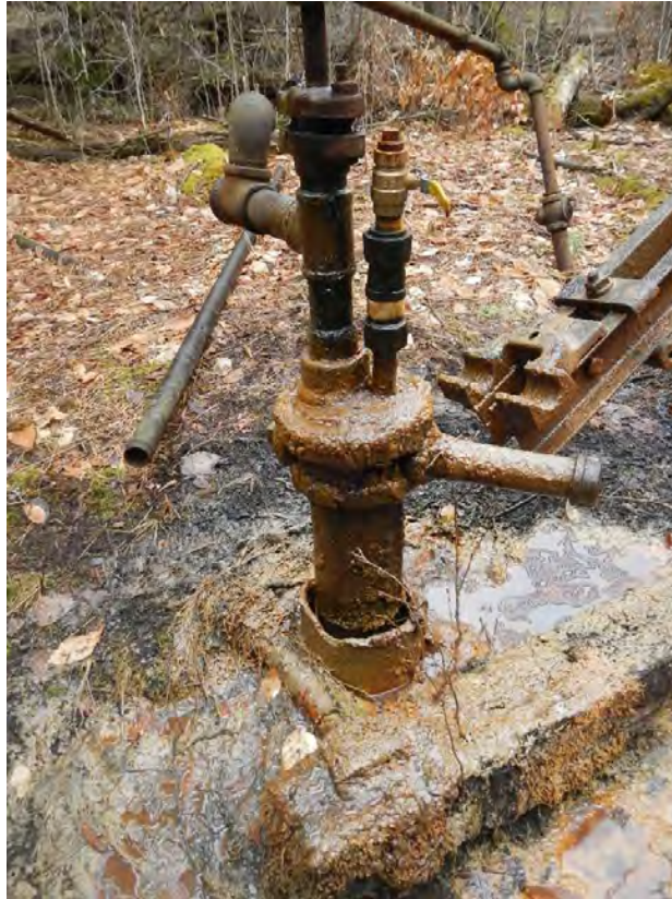
Abandoned Well Oil Spill Next to the Tionesta Creek
