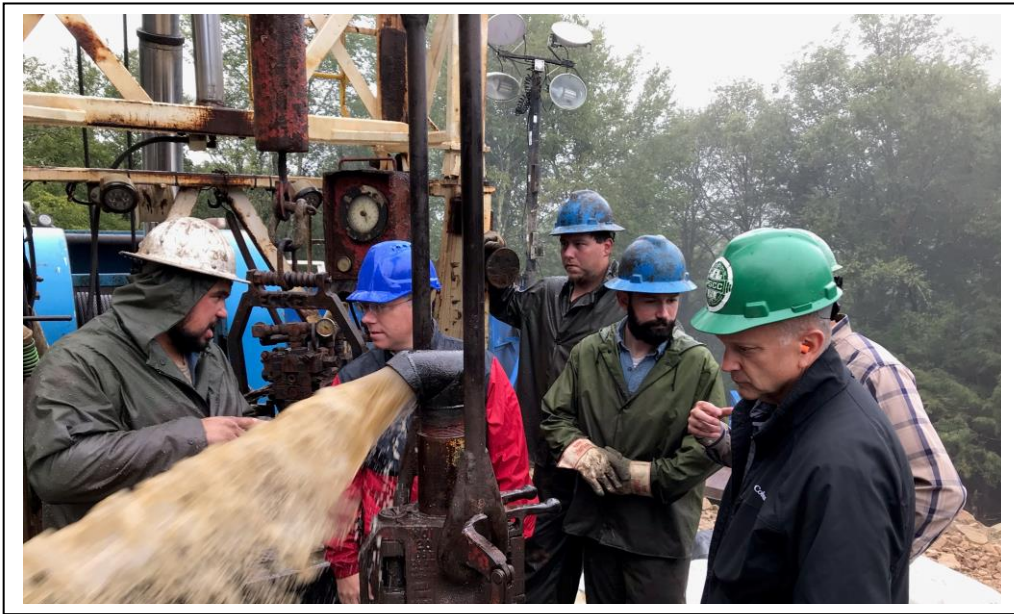
Chairman Metcalfe and Representative David Zimmerman watch the flush from the rig floor
